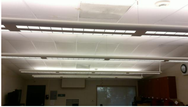
Suspended (2) lamp T8 fixtures in classroom
