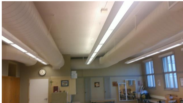
Suspended 2 lamp classroom fixtures
