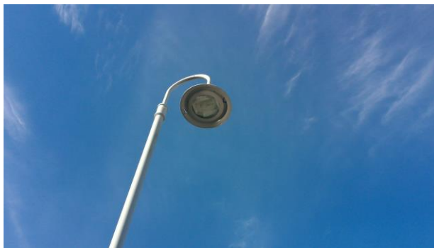
HPS area parking lot fixture
