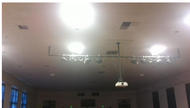
(8) 175 MH surface boxes in auditorium
