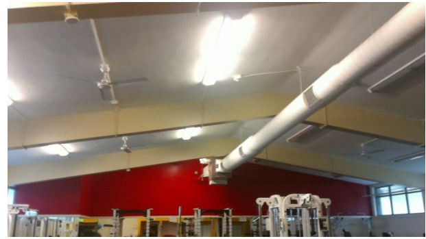
Suspended 2 lamp weight room fixtures
