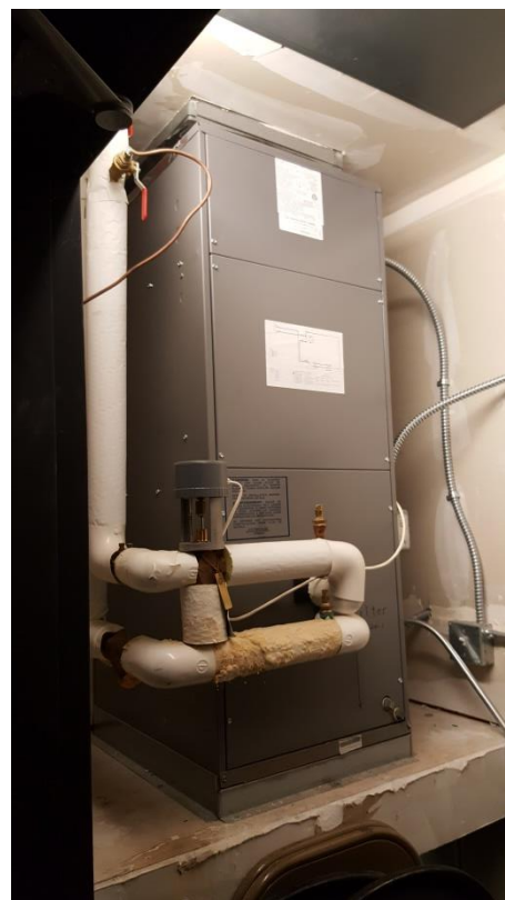
Classroom systems fed from AERCO KC
