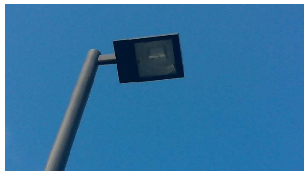
Parking lot area HPR area lights
