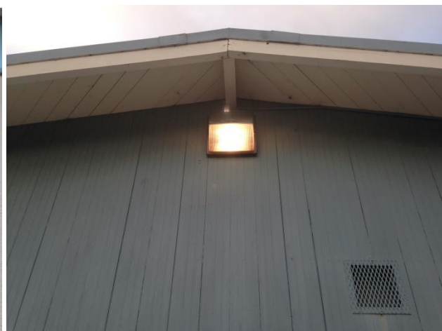
70w HPS wall pack on all day
