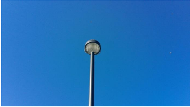
(4) 250w HPS Parking Lot lights
