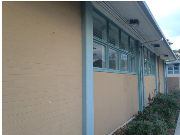
50/70w HPS canopy fixtures
