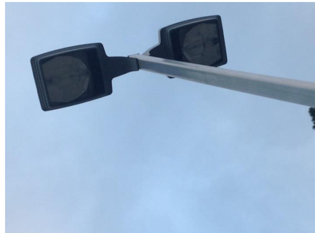
175w metal halide area lights in parking lot
