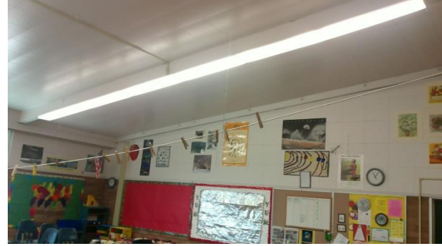
Surface mount 2lamp T8 wraps in classrooms
