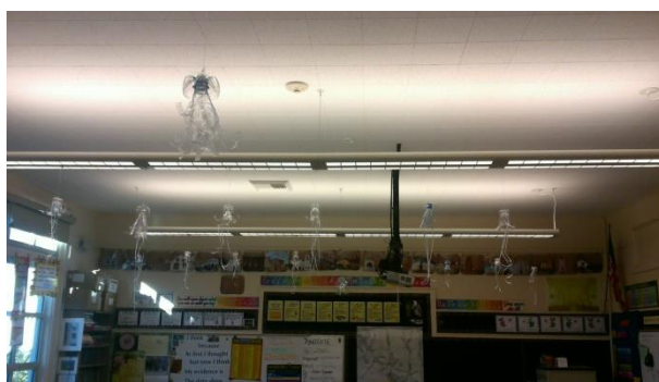
2 and 3 lamp suspended fixtures in classrooms
